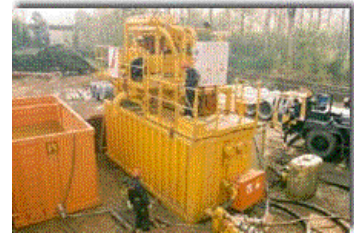
Picture 6: Separation Plant
