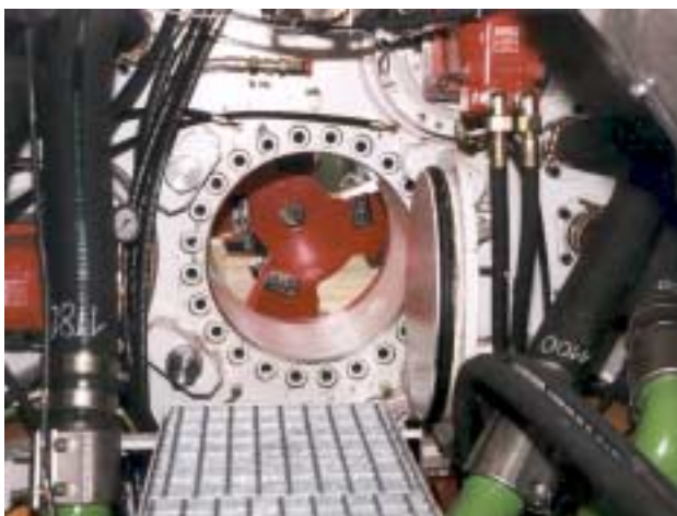
Picture 15: Access hatch
