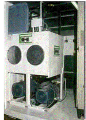
Picture 23: Hydraulic Unit
