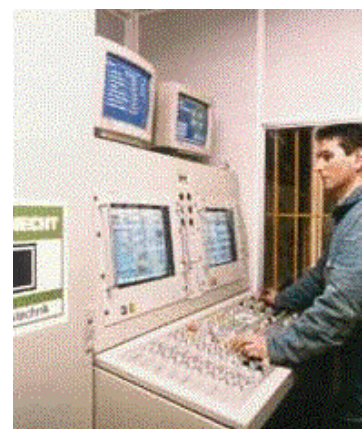
Picture 24: Control Panel
